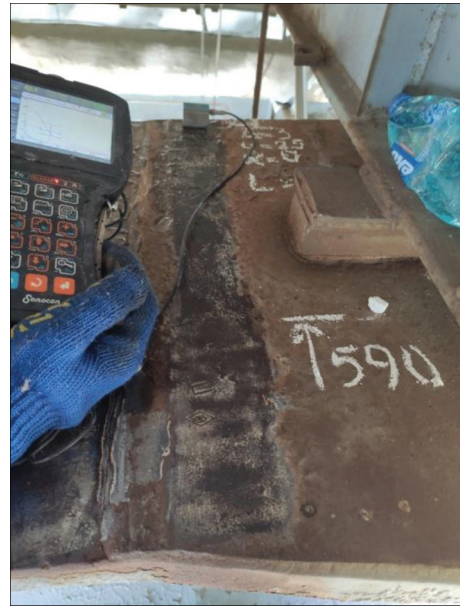
Figure 6. Example of testing butt weld in the upper girth of the joining insert
