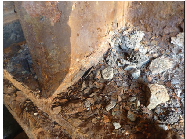
Figure 10. Area of debris accumulation in the supporting part of the four-span structure
