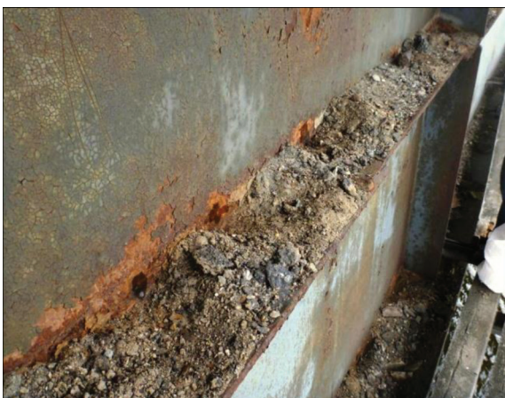
Figure 9. Area of debris accumulation on the outer side of the end beam of the five-span structure
