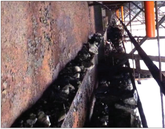
Figure 8. Area of debris accumulation and condition of inspection passages on the inner side of the end beam of the five-span structure
